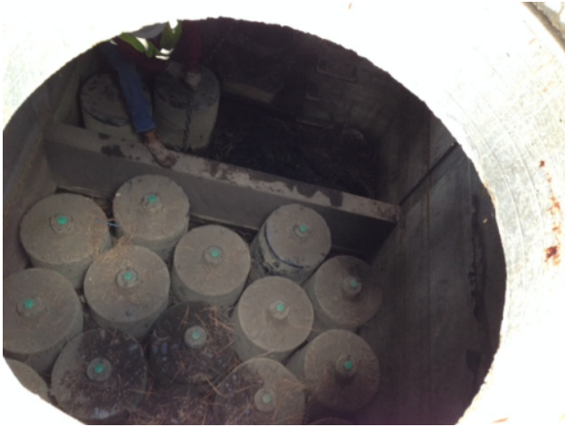
Al Tahoe ECP - Pasadena StormFilter vaults before 2013 cartridge replacement
