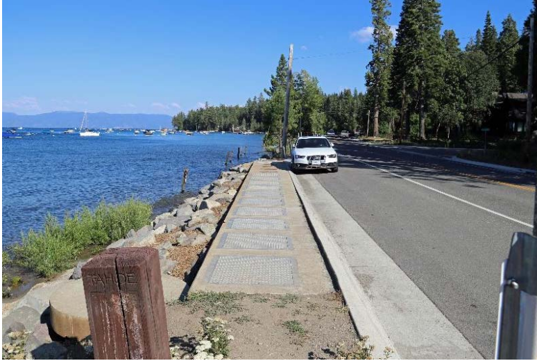
Sand vault treating stormwater before it discharges to Lake Tahoe, constructed as part of the State Route 89 water quality improvement project. (Photo credit: Caltrans)
