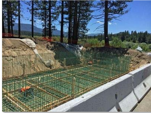
Installation of a Delaware sand filter near the Upper Truckee River in July 2018 as a part of the U.S. Highway 50 "Y" to Trout Creek project (Credit: Caltrans)
