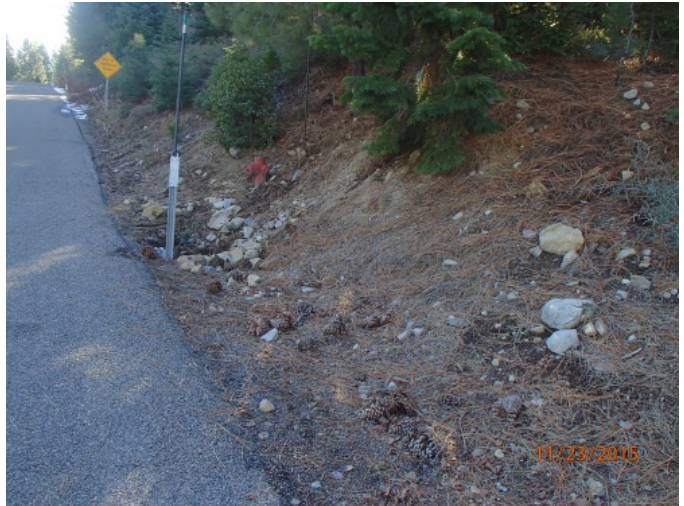
Eroding slope near pipe inlet
