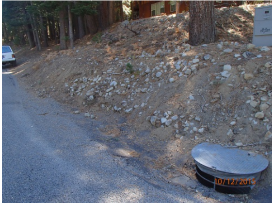
Eroding slope on 10th, at Alder
