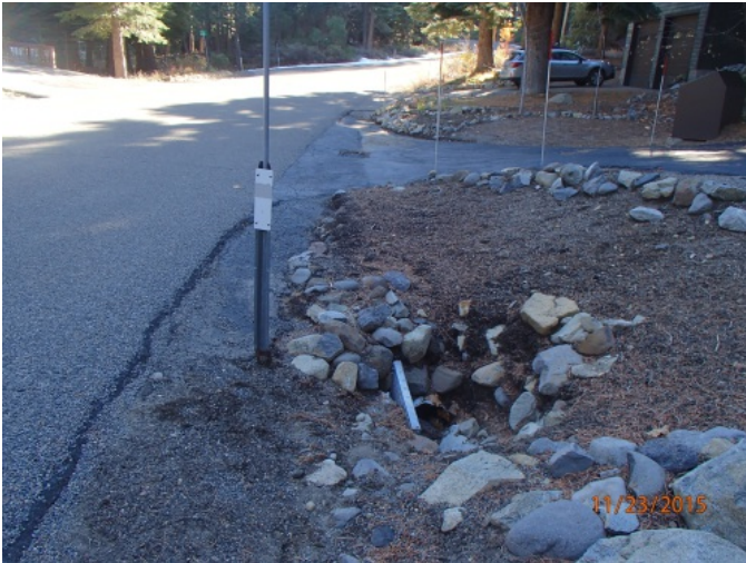
Partially buried pipe inlet(s) on Antelope. Opportunity for Sediment Trap to increase inlet and trapping capacity.
