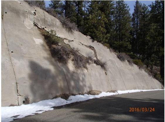
Oflyng - Failing Slope
