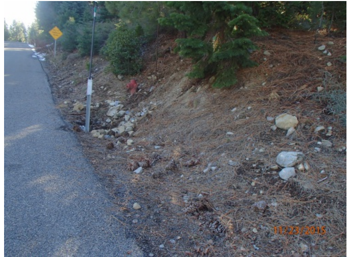
Eroding slope near pipe inlet
