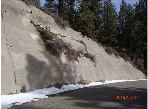
Oflyng - Failing Slope
