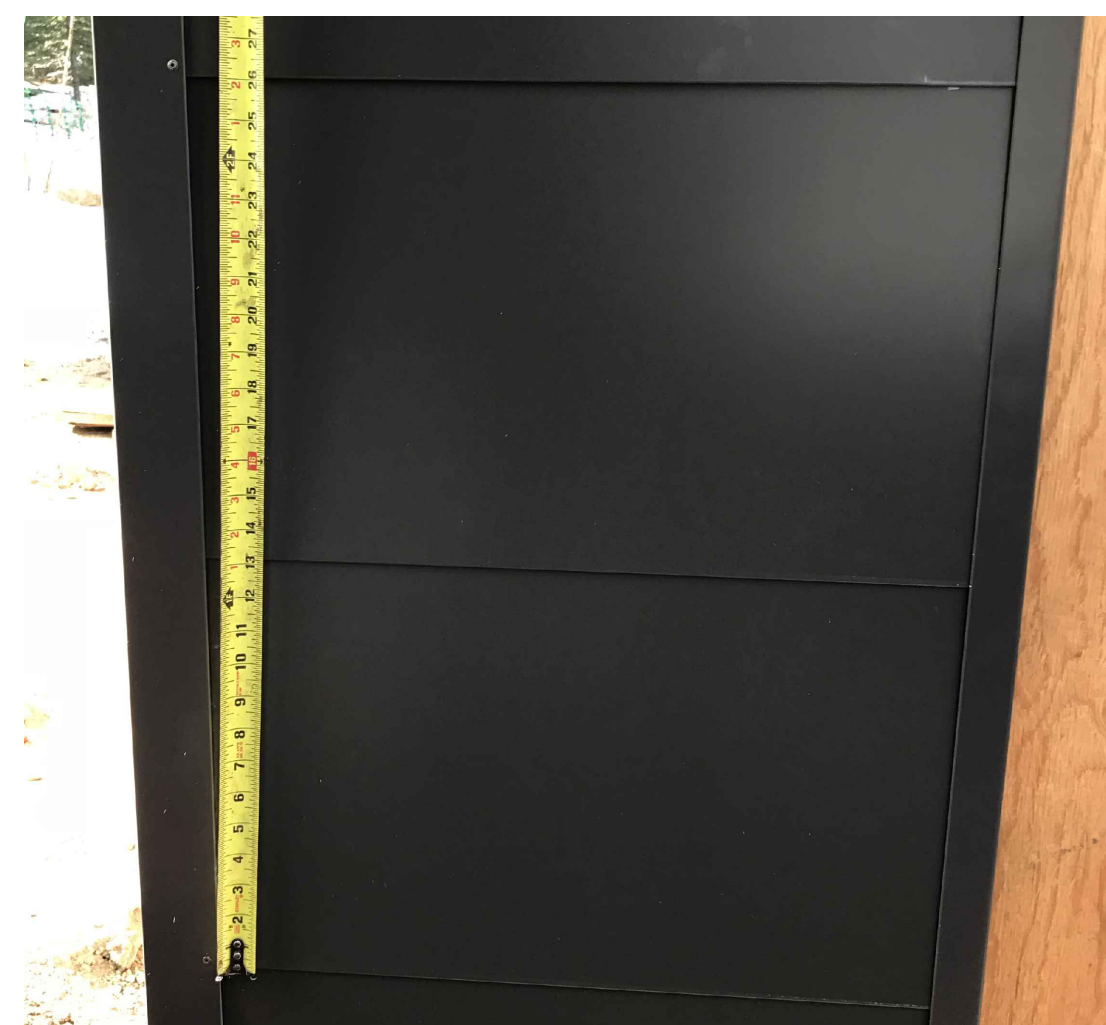
2) METAL PANEL SIDING & TRIM DETAIL. COLOR IS NOT AS PROPOSED - SEE SCHEDULE.
