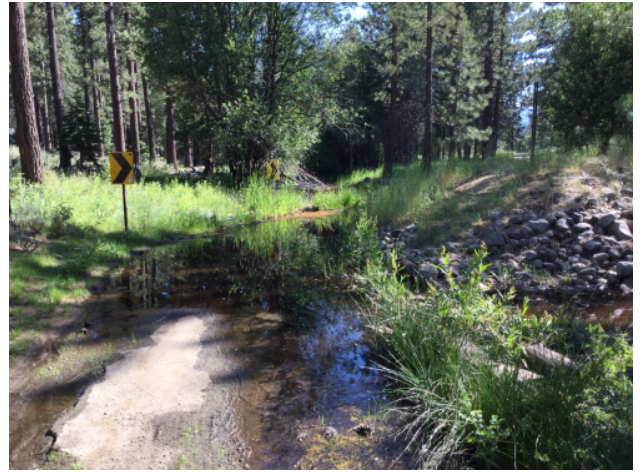
Flooding of existing bike path in SEZ area (July, 2017)
