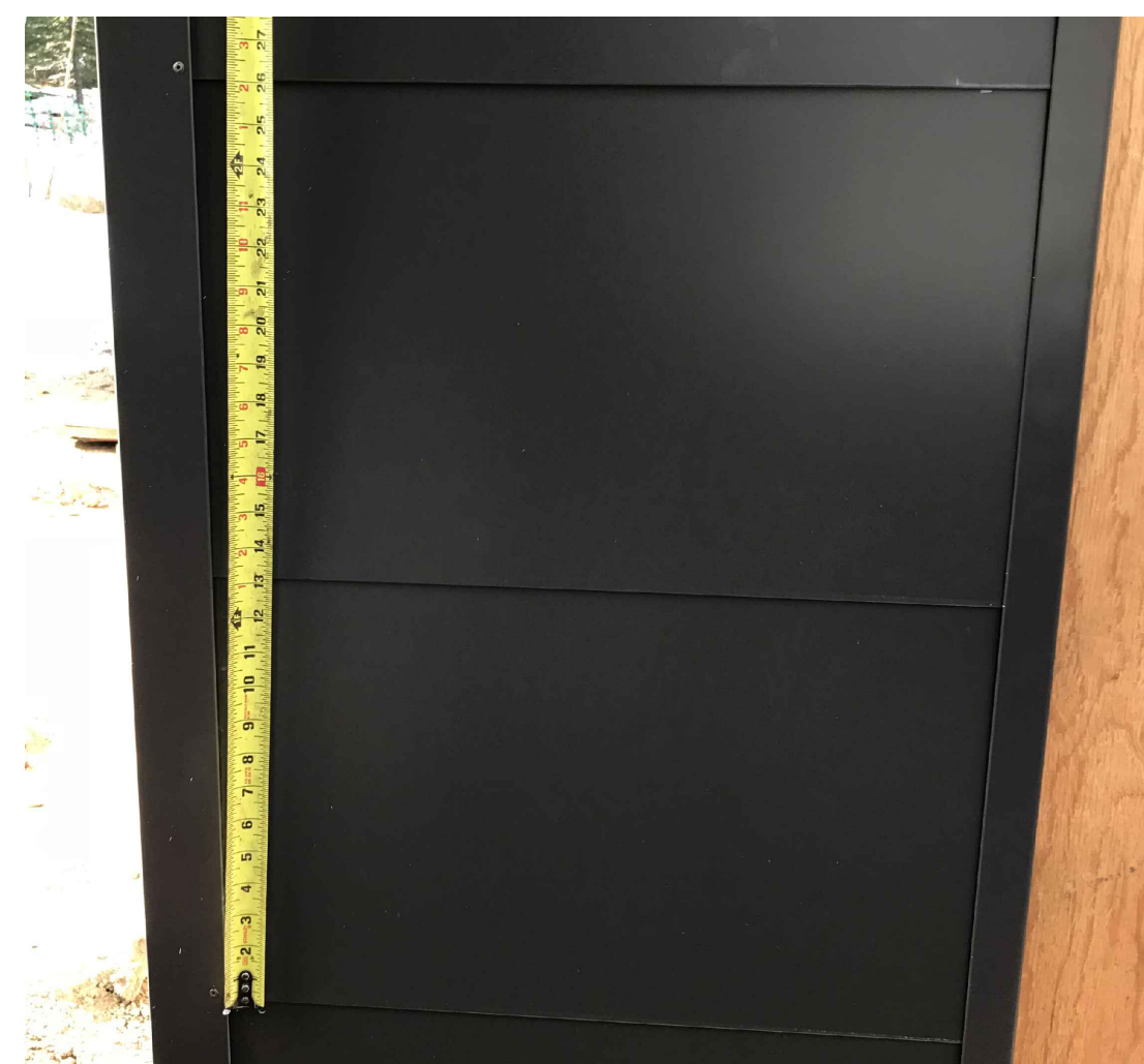
2) METAL PANEL SIDING & TRIM DETAIL. COLOR IS NOT AS PROPOSED - SEE SCHEDULE.
