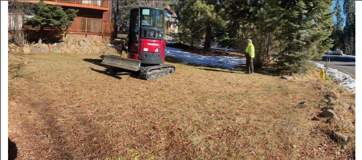
Photo 1 – View south-center of property where mini-excavator is positioning to dig the soil pit. The land surface drops off abruptly (lower right), because it was over-steepened from street construction (circa 1970s). Vegetation consists of Jeffrey pine, white fir, ornamental trees and shrubs, plus lawn.
