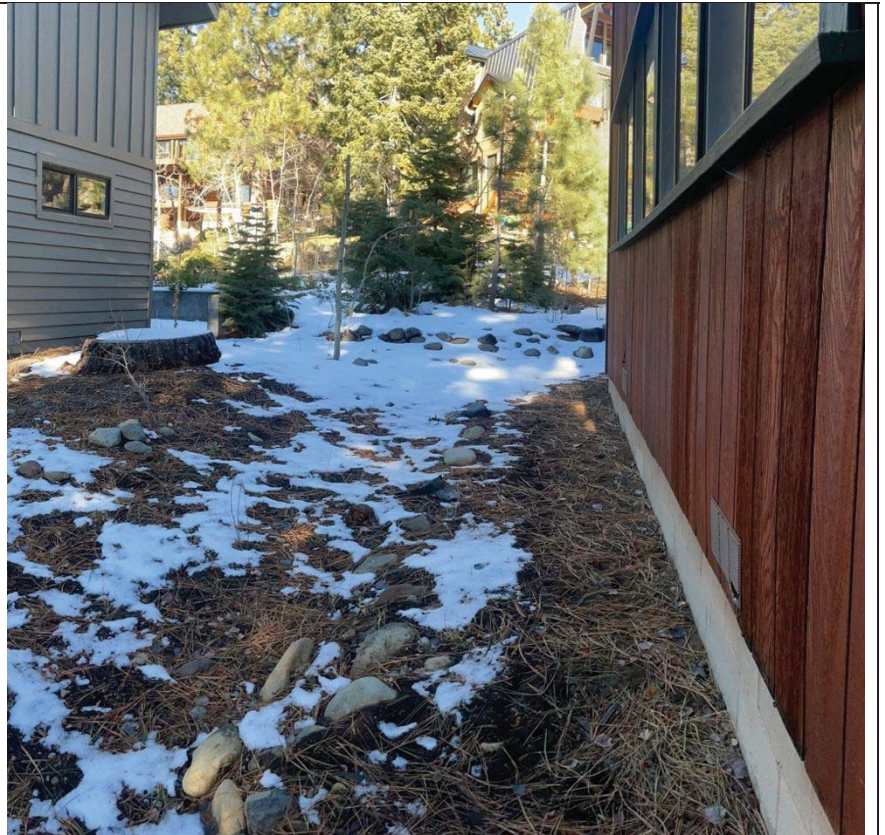
Photo 6 – View west side of residence (reddish brown building at right), where the natural surface appears slightly modified by house construction (circa 1970s) and installation of perimeter BMPs (surface stones in center foreground). For land capability purposes, the natural slopes are relied upon. The slope on this edge of the parcel is 11%. Such slope qualifies this portion of the property as Class 6 for slopes 0 to 16%.
