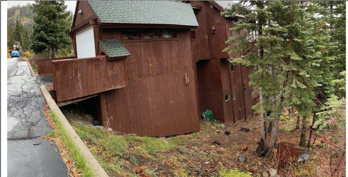
Photo 1 – View east toward residence from west corner of property. Slope immediate downgradient of Verbier Road is artificially steepened. Natural slope on this side of residence is 33%. Tree cover includes white fir, red fir and willow.
