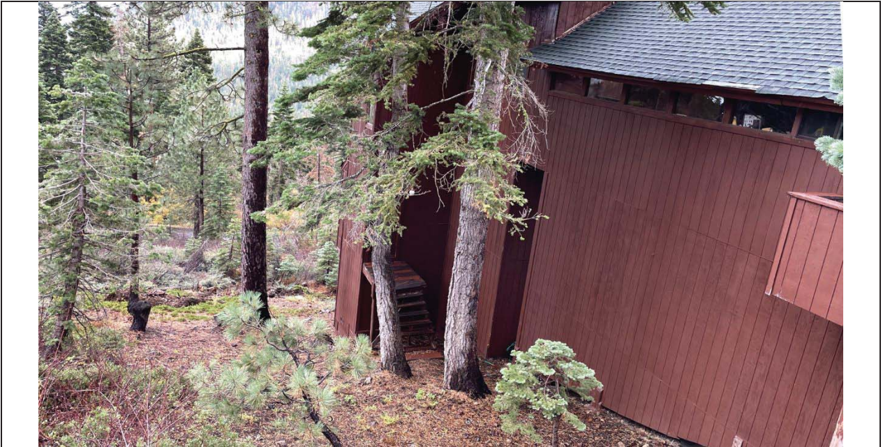
Photo 3 – View to southeast along east side of residence. Ground cover is good with 25 to 35% vegetation and 65 to 75% fir needles, twigs, and leaves. No indication of active erosion.
