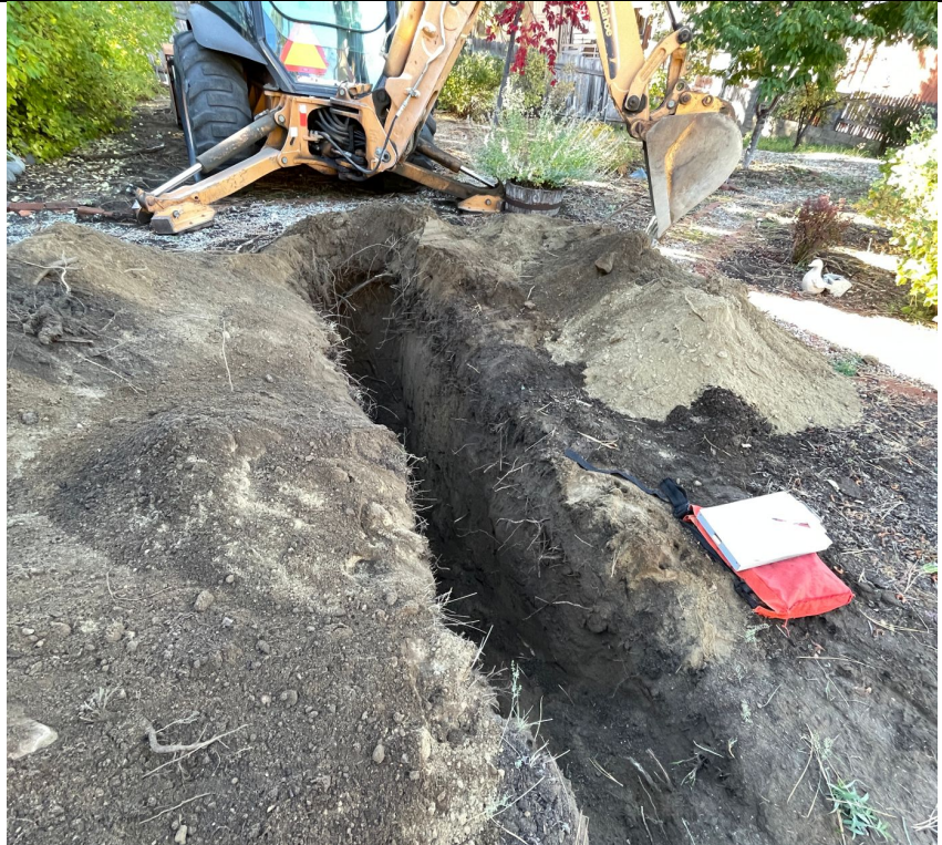
Photo 2. View south at Soil Pit no. 1. Roots extended to bottom of soil pit with no indication of seasonal high water.
